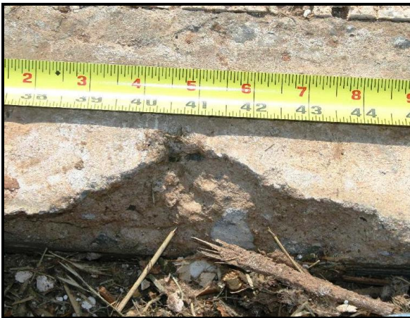
Figure 5. Broken edge of the concrete slab foundation where a perimeter wall plate had been secured with a cut nail.
