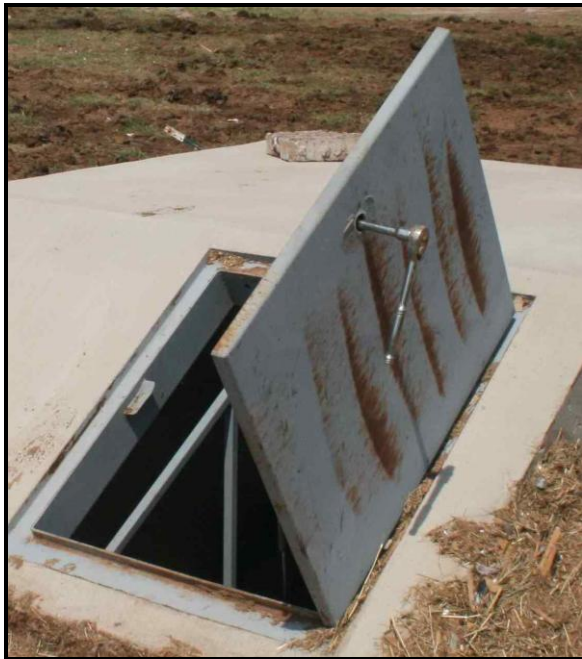
Figure 8. A partially below grade storm shelter had lost its door handle. A wrench was used to open the door.
