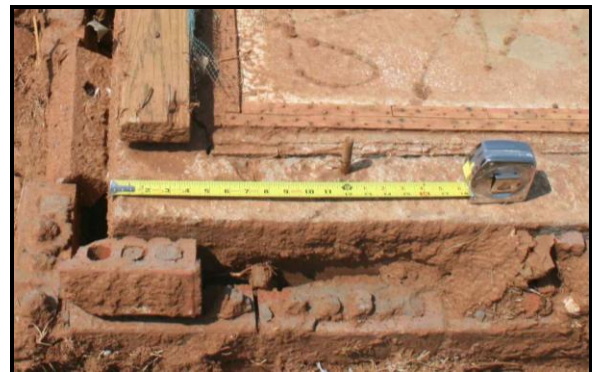
Figure 13. Close up view of southwest corner of concrete slab foundation. Anchor bolts were missing nuts and washers.
