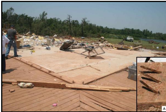
Figure 19. A leveled one- and two-story home at 212 th Street and Cedar Lane: a) wall failure occurred when straight-nailed connections pulled apart.
