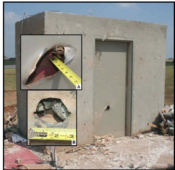
Figure 10. A cast-in-place, steel reinforced concrete shelter survived the tornado but had a damaged door: a) outer panel penetration, and b) damaged deadbolt lock mechanism.
