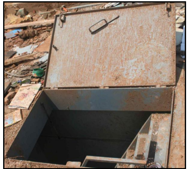
Figure 22. Occupants survived in this below ground storm shelter but were trapped when a vehicle slid over the door during the tornado.
