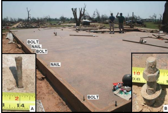
Figure 17. A single-story house at Rockwell Road and Highway 76 was swept clean from its concrete slab foundation. Perimeter wall plates were secured with alternating: a) cut nails and b) anchor bolts.
