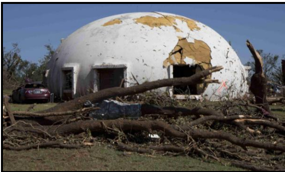
Figure 16. A fiber and steel-reinforced concrete dome home survived a direct hit by the tornado.
