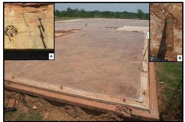
Figure 21. This house was swept clean from its concrete foundation on Highway 74B just west of High Road: a) wall failure occurred at straight nailed connections, and b) not all anchor bolts had nuts and washers.
