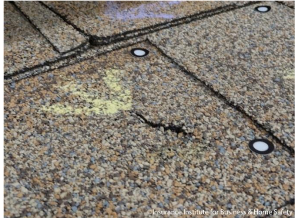
Figure 12: A tear, crack, or rupture is a 1D measurement expressed as a length.
