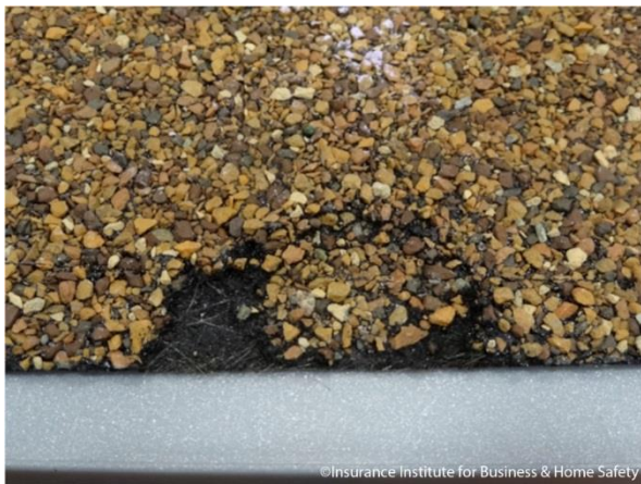
Figure 10: Clusters of granules missing that result in exposed asphalt and/or fibers are known as “patch granule loss”. These 2D measurements are expressed as an area.
