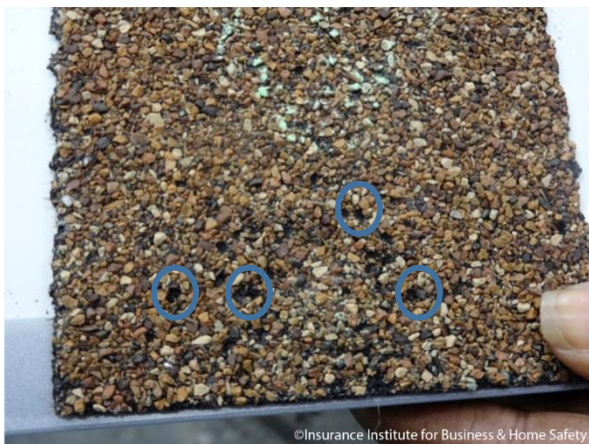
Figure 11: Single or many granules missing that are not clustered and give a pitted appearance to the shingle surface are known as “individual granule loss”. These 2D measurements are expressed as an area.
