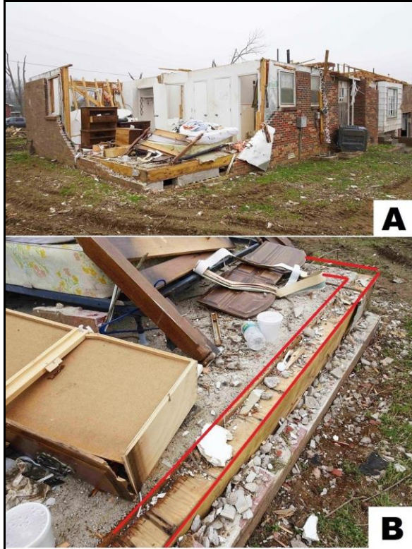
Fig. 3. Damaged home due to the tornado: A) loss of roof and a portion of the exterior frame wall, and B) failure point was where frame walls were attached to the floor (outlined in red).
