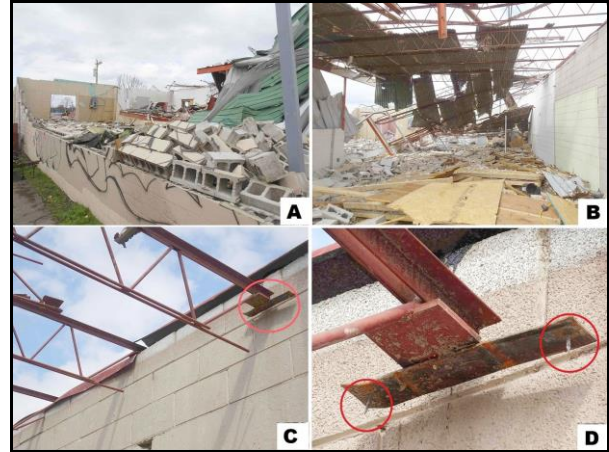
Fig 8. Damage to a strip mall: A) toppling of the southwest unreinforced masonry wall, B) loss of roof decking, C) steel joist hanging off wall, and D) nails (circled) in steel plate had pulled out of wood nailer secured to the top of the CMU wall.
