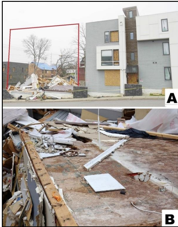
Fig. 5. Part of a three-story apartment building that collapsed: A) outline of building, and B) closer view showing floor platform where base of wall was straight nailed.
