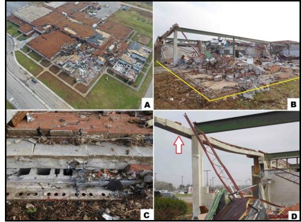
Fig.12. Damage to West Wilson Middle School. A) Drone image looking east, B) destruction of southwest classrooms, C) base of masonry wall toppled inward, and D) bond beams (arrow) hanging between supports.
