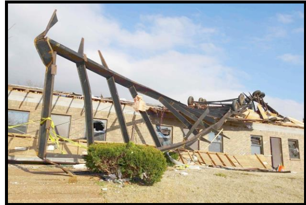
Fig. 4. Steel frame of unanchored manufactured home deposited on the Donelson Christian Academy.
