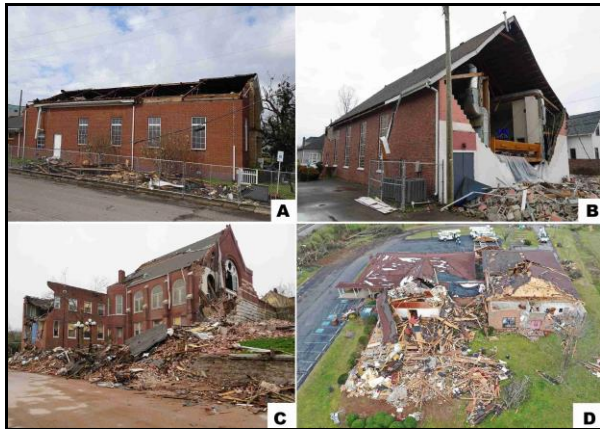
Fig. 19. Various degrees of damage to churches: A) loss of roof, B) toppled end wall, C) toppled bell tower and brick façade, and D) collapse of sanctuary.
