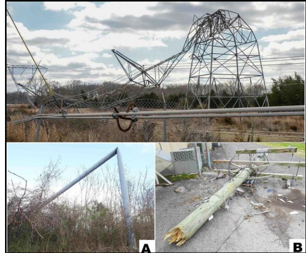
Fig 16. Damage to electrical transmission systems: A) toppled steel truss tower, B) bent tapered steel pole, and C) broken wood pole.
