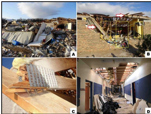
Fig 9. Damage to Donelson Christian Academy: A) collapse of south wing, B) masonry wall collapse around doors and windows (yellow outlines) with bond beams remaining (arrows), C) toe nailed roof truss, and D) interior hallway.
