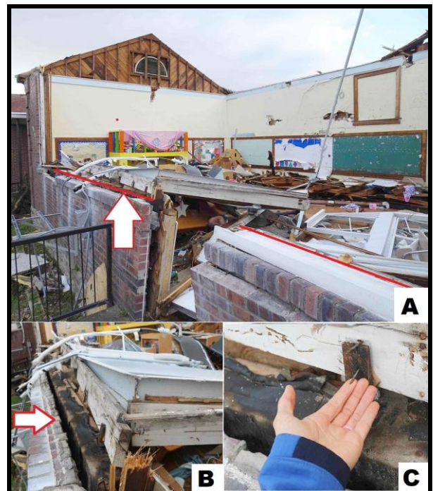
Fig. 10. Damage to classroom at the Dodson Chapel United Methodist Childcare: A) windows toppled inward at hinge line (red line and arrow), B) closer view showing wood nailer (arrow), and C) nails pulled out of wood window frame.
