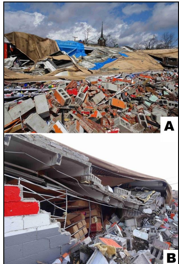
Fig. 6. Collapse of Auto Zone store: A) unreinforced, loadbearing, masonry walls, and B) heavy concrete tee roof deck.
