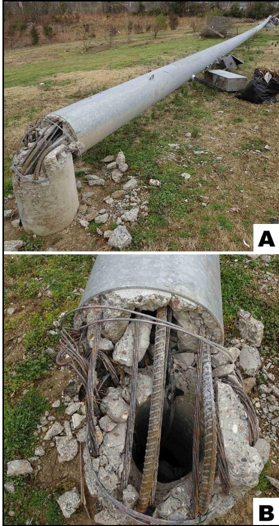
Fig. 17. Broken pier cap which supported tapered steel light pole: A) overall view, and B) close-up view of broken concrete pier.
