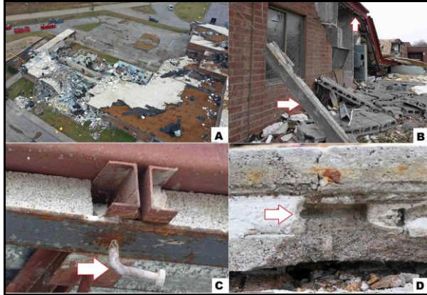
Fig. 13. Damage to Stoner Creek Elementary: A) collapse of CMU walls and roof due to poor attachments, B) lack of bond beam (horizontal arrow) attachment to wall, C) bent pegs at roof that were merely set into mortar channel along D) tops of bond beams.
