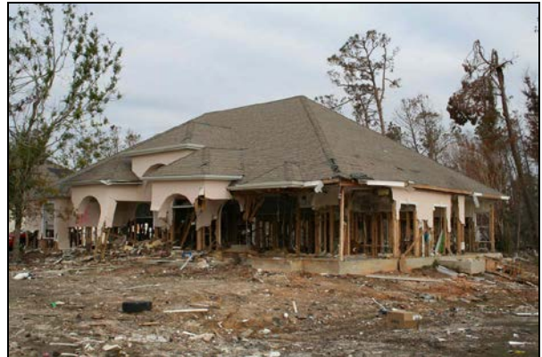
Figure 8. Moving water gutted this wood-framed house on a slab foundation in Long Beach, MS. There was minimal wind-caused damage to the roof shingles.
