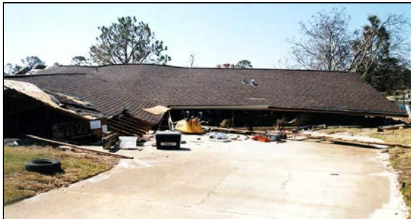
Figure 6. Walls collapsed when this house became submerged in Pensacola, FL leaving the roof upright on the foundation.
