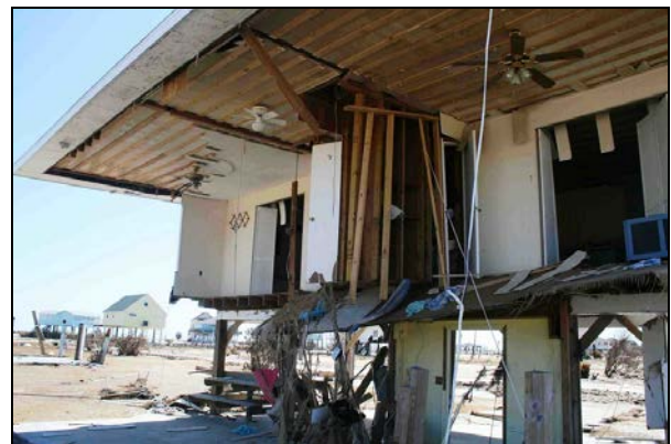
Figure 13. Wave action undermined and removed the floor structure on this elevated wood-framed house on the Bolivar peninsula. Note ceiling fans remained intact.
