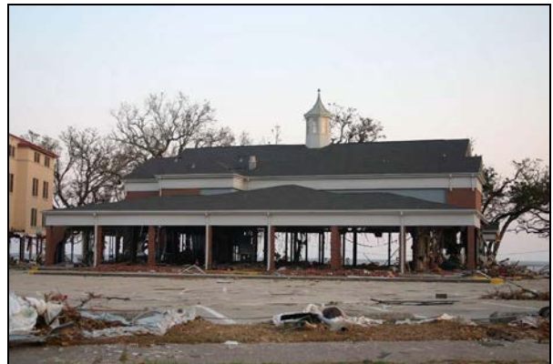
Figure 16. The first story of this steel-framed building was gutted by storm surge in Gulfport, MS. There was no wind damage to the roof covering including the cupola.
