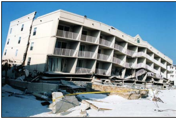
Figure 18. Catastrophic collapse of what was a five-story concrete-framed building in Orange Beach, AL. Waves removed the load bearing walls.
