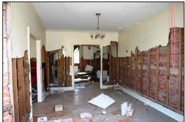
Figure 9. Wave action and floating debris removed the gypsum board sheathing inside this home, not wind. Note the chandelier remained undamaged.
