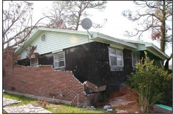
Figure 4. This wood-framed home in Pass Christian, MS floated within the broken brick veneer shell but did not come back to the same position. This condition was not caused by wind. Note wind did not damage the gable siding or satellite dish.
