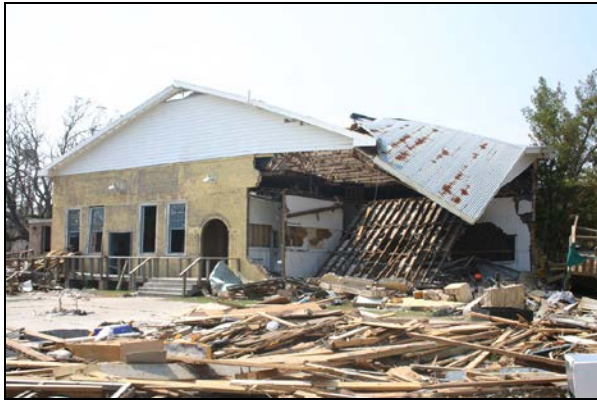
Figure 14. Partial collapse of masonry walls due to moving water and repeated impacts of floating debris in Waveland, MS. There was a 3m water line above the floor inside this building.
