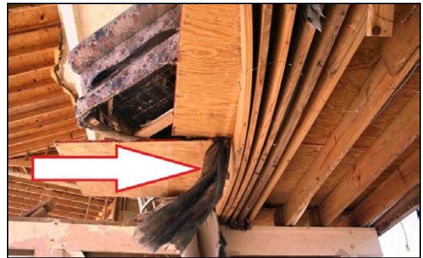
Figure 12. Progressive stacking of floor joists towards the landward side of the building due to the force of moving water and wave action (arrow).
