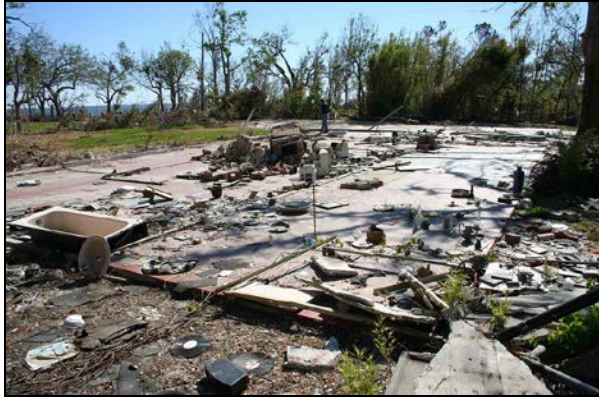
Figure 10. Storm surge removed the entire building from the property, leaving only heavy items. Unbroken glass items remained on the slab indicating the building was dismantled slowly.
