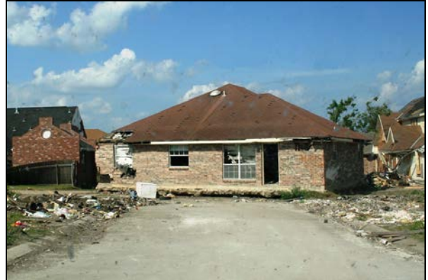
Figure 7. This wood-framed home floated along with its concrete slab foundation in Meraux, LA. Buoyancy forces overcame the weight of the building assembly. Wind did not lift the building.
