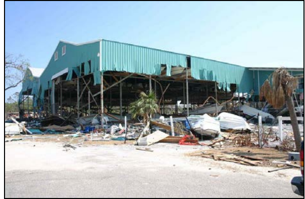
Figure 15. Removal of metal wall cladding and girts due to moving water and repeated impacts of floating debris. This building was in Pass Christian, MS.
