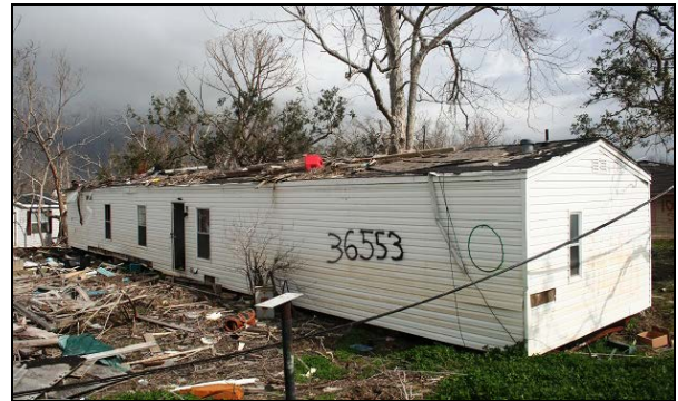
Figure 2. This manufactured home was moved off its foundation by moving water (not wind) and was stopped by a tree in Venice, LA. Note flotsam and floating debris on the roof as well as the absence of wind-displaced siding.
