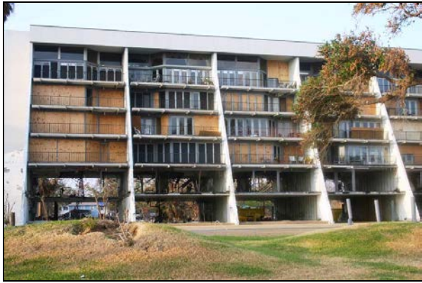
Figure 17. Moving water removed the interior partitions and contents in the lowest stories of this building in Biloxi, MS.
