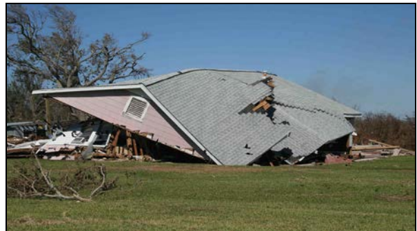
Figure 5. This wood-framed house was undercut by moving water and debris in Bay St. Louis, MS. The house has the typical “pitched-down” appearance toward the water. Note the absence of wind damage to the roof shingles.
