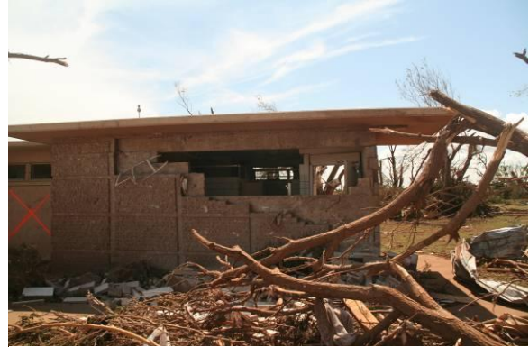
Figure 5: Remains of a concrete bathhouse which sheltered approximately 10 individuals during the tornado.
