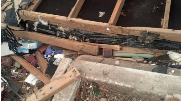
Figure 10: A close up of a home's base-plate-to-foundation connection. Shot pins were used to secure the base plate to the connection, with bolts not even being used in the corners.
