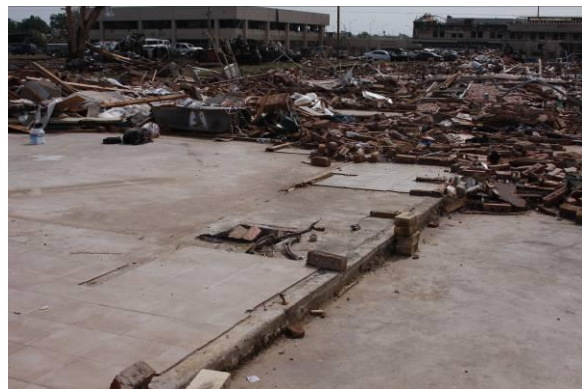
Figure 11: One of 4 homes assigned an EF5 rating near Moore Medical Center. All four homes were swept from their foundations, with removal of base plates and bent anchor bolts. The resident of this home was injured sheltering from the tornado in the bathtub.
