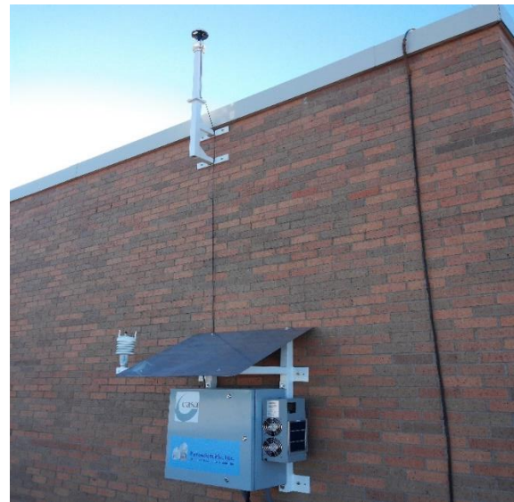
Figure 5. Physical installation on top of Nedderman hall, University of Texas Arlington.
