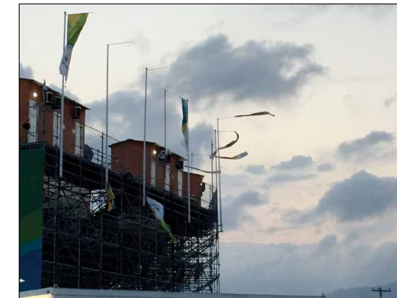
Minor damage to the spectator grandstands after the Aug 15 wind event. Mesh was ripped from the scaffolding and the grandstand flags were ripped and tattered.
