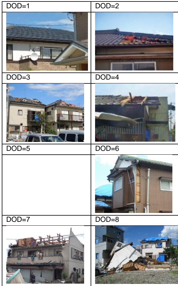
Fig. 4: Example damage cases of each DOD in DI=1 “Wooden houses or stores.” There is no photo for DOD=5 available.
