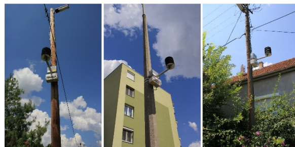
Figure 2. Typical setup of monitoring stations
