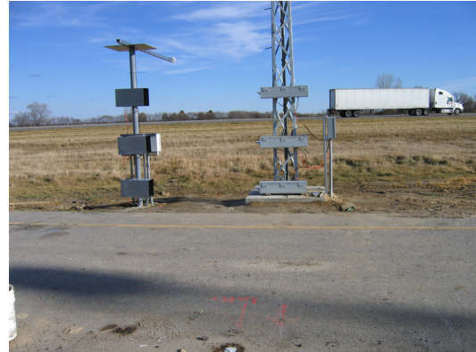
Fig 3: The grey boxes mounted on the left pole house the light sources. The grey boxes located on the tower hold the camera enclosures. The reason for the enclosures is to ensure security to both the lights and cameras. I-29 is the highway in the background and the road in the foreground is the access road to the abandon rest stop.
