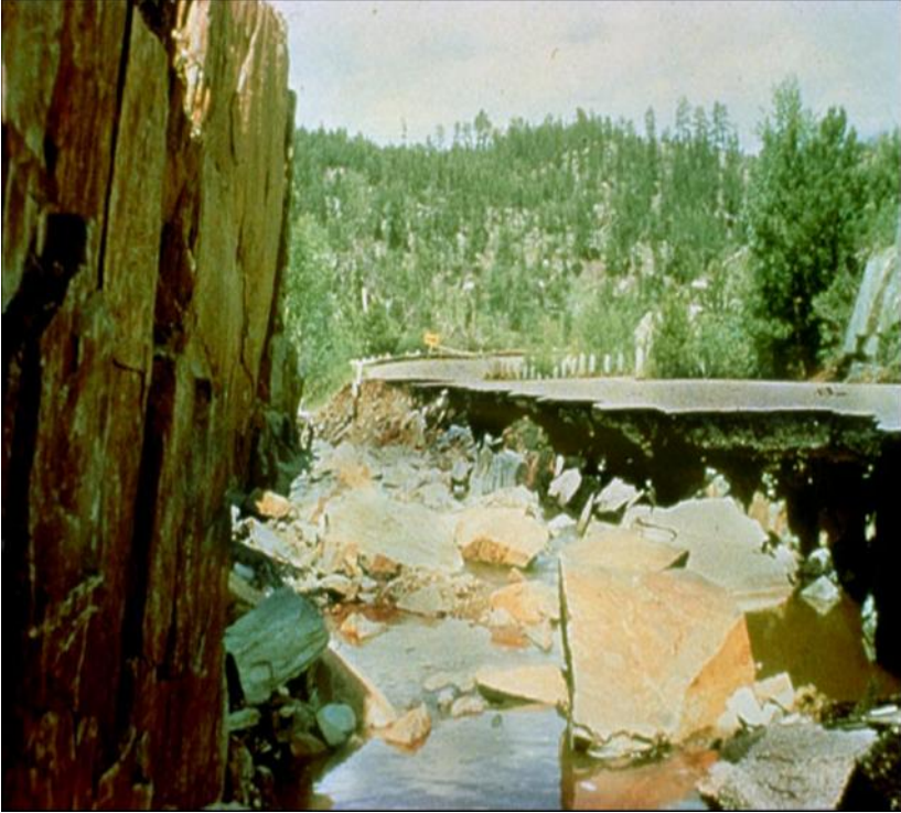
Figure 5: Damage to U.S. Highway 34 in the Big Thompson Canyon, Colorado from the 31 July 1976 flash flood.
