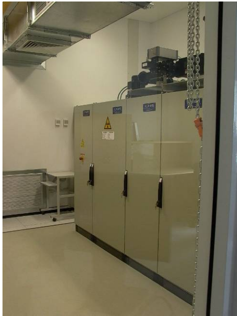
Figure 3 – Radar Equipment Room
