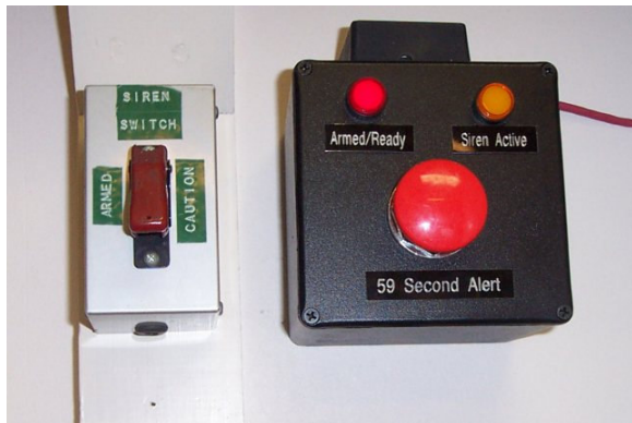
Figure 10. Control panels for tornado siren in Dallas/Fort Worth, Texas. (courtesy bensware.com)
