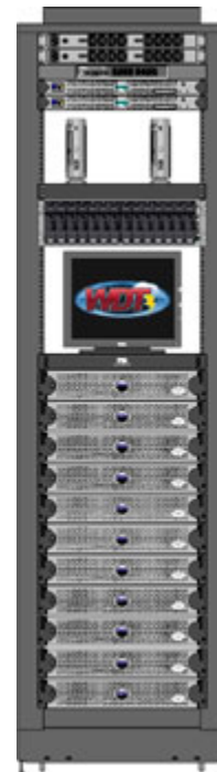
Figure 4 AWDSS Hardware Rack
