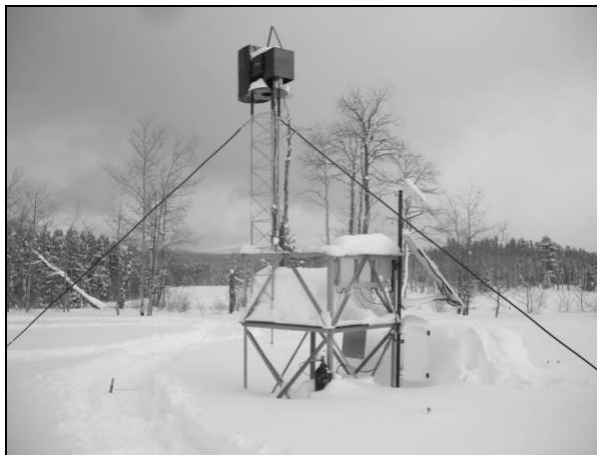
Figure 1. A WMI remote-controlled generator is shown mid-season, January 2008. Buried beneath the snow are the propane and seeding solution tanks. The "triangle" atop the burner housing is a "perch guard", installed to discourage raptor nesting. Also below the snow is fencing to keep grazing animals away from the unit during the summer months. The total height of the assembly is 7.6 m (25 ft).
