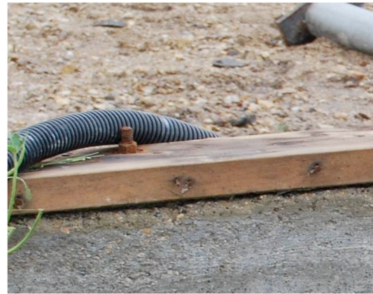
Figure 2. Sill plate with anchor bolt still attached to the foundation on House #1.
