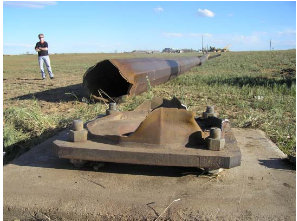
Figure 2. Power line support sheared off at base. Estimated winds 140 mph -155 mph. Evaluated as EF3. Location is near the Missile Silo Park Campground west of Greeley. (Courtesy NWS BOU)
