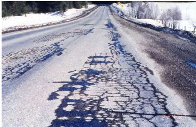
Figure 3 – Road damage caused by frost heave (Credit: Washington State DOT)
