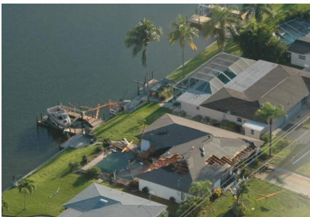
Fig 1. Cape Coral tornado damage, 16 September 2007.
