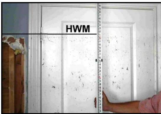
Figure 3. Example of a high water mark on the interior of a building.
