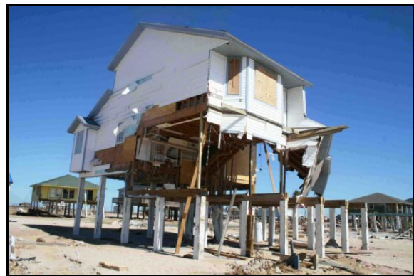
Figure 5. This home lost most of its first elevated floor and several walls due to wave action but, remarkably, did not collapse. By contrast, houses farther inland (in background) were not damaged since wave action was less severe.
