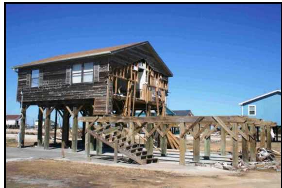
Figure 6. Storm surge removed the lower portion of this home leaving the upper portion intact. Generally, buildings at low elevations were susceptible to being damaged or destroyed by storm surge and wave action.
