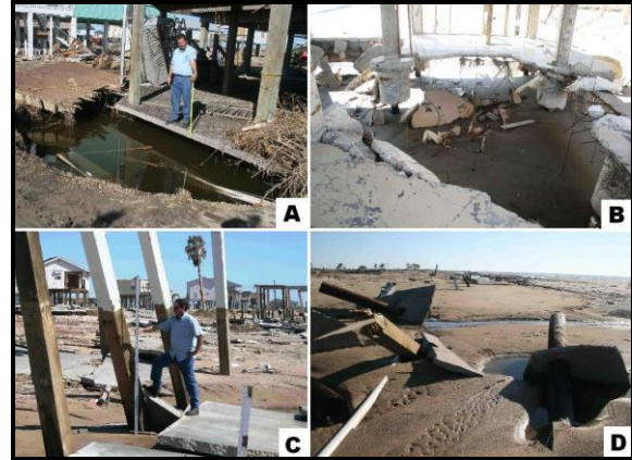
Figure 8. Increasing degrees of damage to foundations of elevated wood-framed residences in the scour zone: a) partial scouring of sand beneath slab on grade, b) complete scouring of sand and collapse of slab on grade, c) removal of slab on grade and leaning of the pilings, and d) total loss of piling support.
