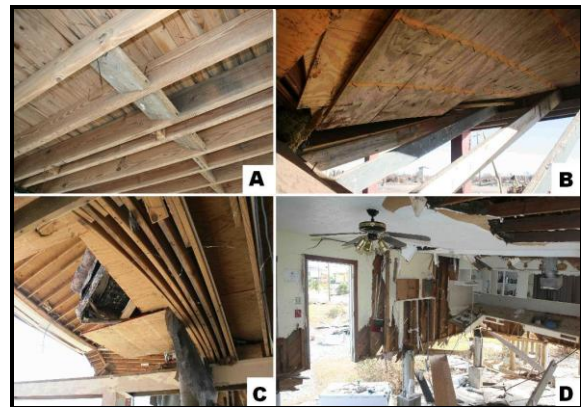
Figure 9. Increasing degrees of damage to flooring on elevated wood-framed residences: a) rotation of blocking, b) uplift of flooring, c) landward stacking of floor joists, and d) complete loss of the floor structure.
