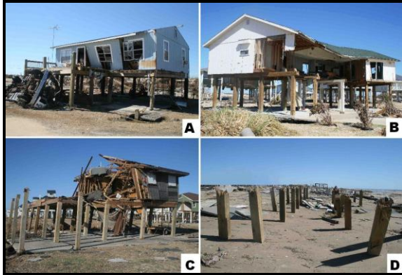
Figure 10. Increasing degrees of damage to elevated wood-framed residences in Hurricane Ike: a) damage to a seaward wall, b) loss of seaward walls and part of the floor, c) partial collapse of a house, and d) completely destroyed house with only timber piles remaining.
