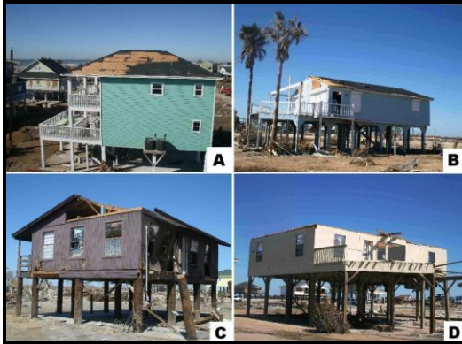
Figure 12. Increasing degrees of wind damage to elevated wood-framed residences in Hurricane Ike: a) loss of roof shingles, b) loss of a porch covering, c) partial loss of the roof structure, and d) total loss of the roof structure.
