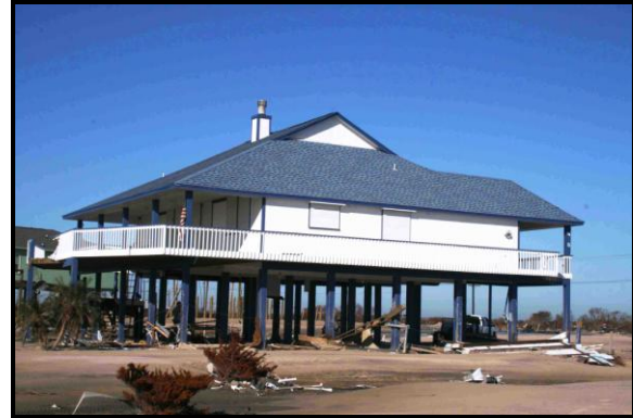
Figure 11. A well-built house that survived Hurricane Ike was elevated above the level of the storm surge and wave action. Also, the home was located inland, with no scouring around the pilings.
