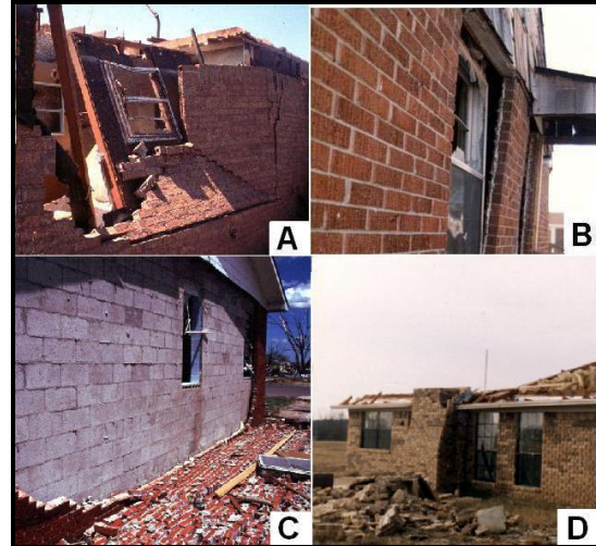
Figure 3. Failure of masonry in the wind: A) windward wall toppled inward around a window, B) leeward wall leaned outward around a window, C) toppled wall along a hinge line at the base of the wall, and D) a broken chimney at roof level.
