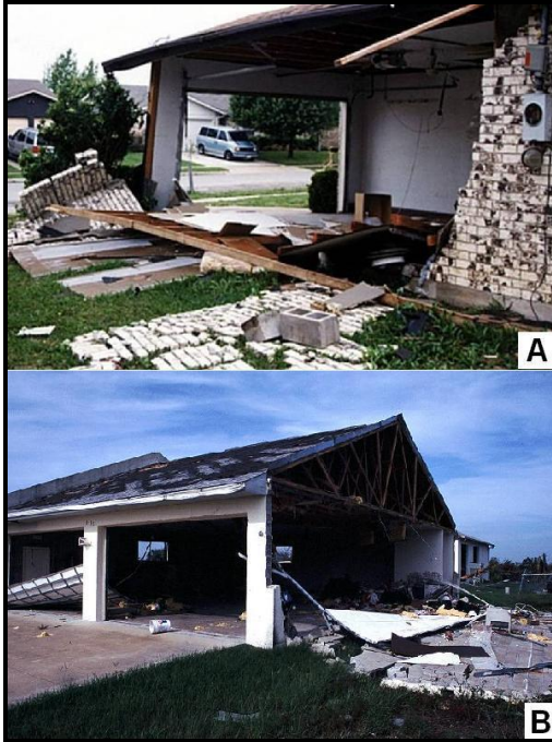
Figure 2. Failure of the garage doors led to internal pressures that helped topple the: A) brick wall and B) concrete masonry unit wall.
