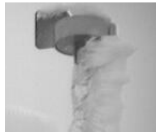
Fig. 3. Icing on the Hydro-Tech direction vane and mast.
