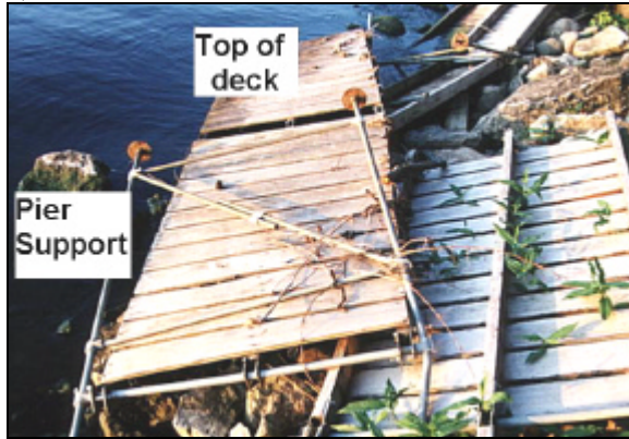
Figure 5. Boat pier debris on the shore of Lake Butte des Morts after the storm.
