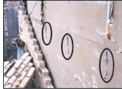
Figure 7. Brick ties (circled) were not bent into mortar joint, so the brick wall was not attached to the house.
