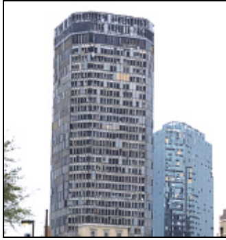
Figure 5. West façade of the Bank One Tower (left) and the UPR building (right) showing extensive loss of window glass.
