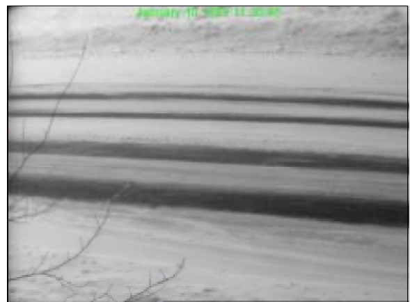
Figure 8. Photograph of the test location showing wide variation in pavement conditions across the road
