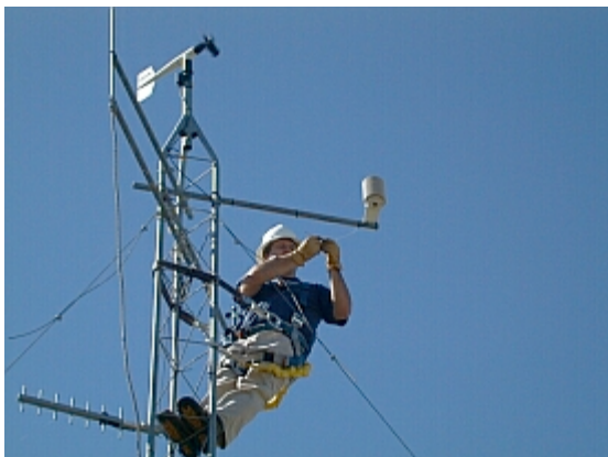
FIG. 3. Mesonet technician inspecting and cleaning sensors at the 9 m level.
