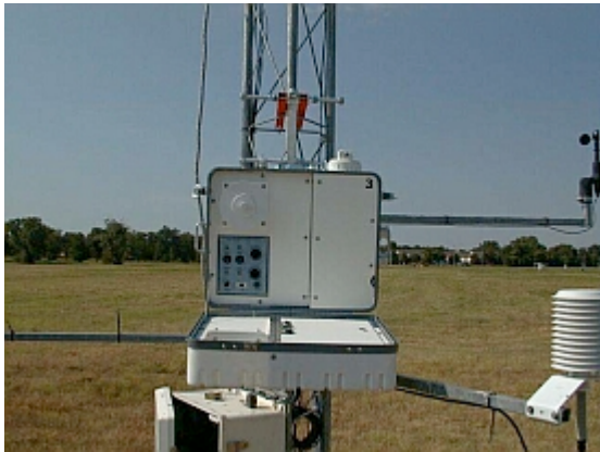
FIG. 5. Portable reference system used to verify field performance of various sensors.
