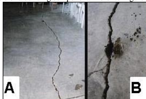
Figure 2. Old crack in middle of concrete slab (A) and close-up view (B) showing dirt in crack. This crack was not caused by the hurricane.
