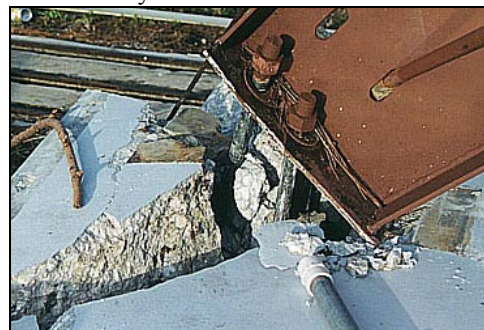
Figure 3. New crack in concrete slab caused by the rotation of the steel column that failed in the wind.
