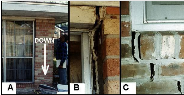
Figure 4. Foundation settlement at the corner of a house (A). Close-up view (B) shows V-shaped gap between window and brick, and (C) shows stair-step crack at base of window. Note prior attempts at caulk repair. The distress was not caused by the hurricane.
