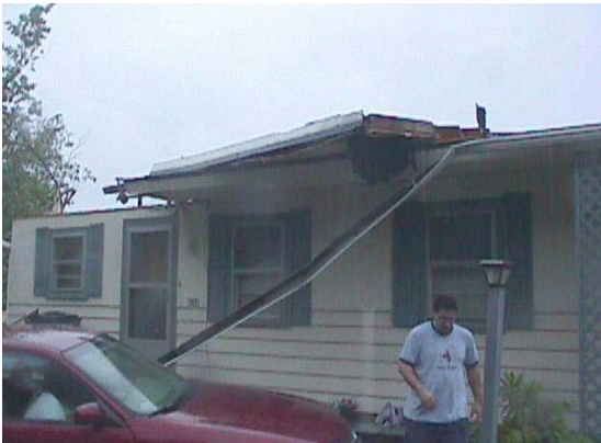
Figure 5. Roof blown off house adjacent to Lake Wickaboag. Photo by Glenn Field.
