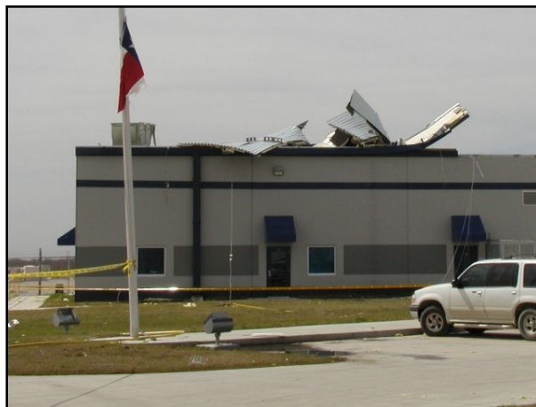
Fig. 11. Tornado damage to a warehouse building in southern Ellis County near Ennis, TX. The convective cell associated with the tornado is depicted in Fig.7.
