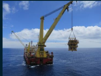
Going one step further is forecasting the crane boom motion and then the movement of the load throughout a lift.
